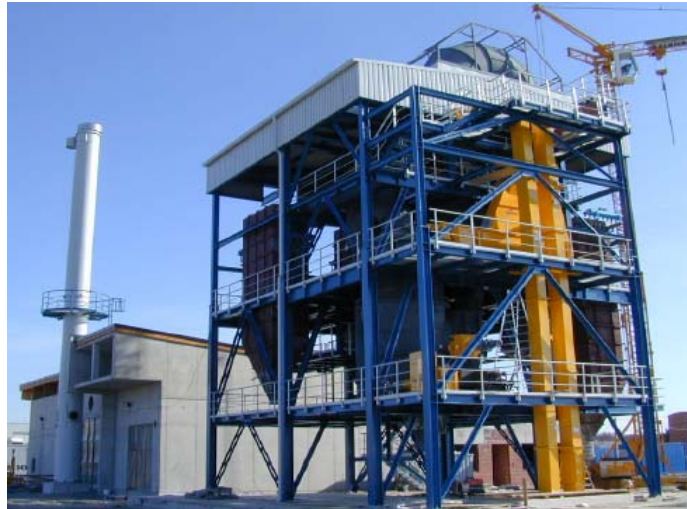
Figure 40 The CHP plant in Güssing, Austria
